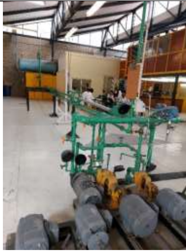
Fig. 6. Sliding train of centrifugal pumps
