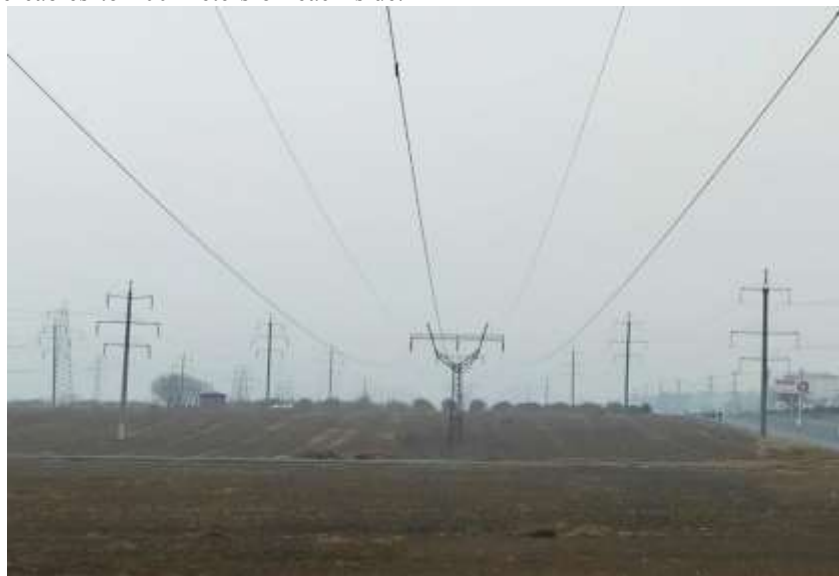
Picture-1 Parallel air power lines in the city of Fergana, Sh.Rashidova Street (transverse view)
