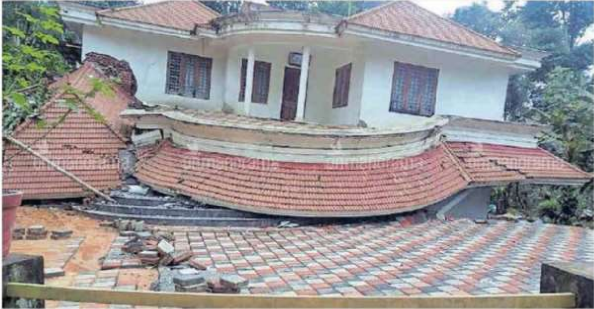
Fig.3. House that sunk into earth (Manorama online, 2018)
