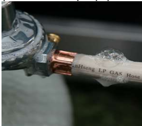
Fig 1.a LPG Leaking out
