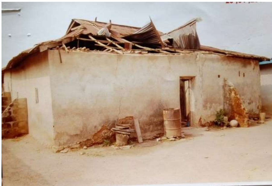
Source Author Fieldwork 2018 Plate1 Building affected by Rainstorm
