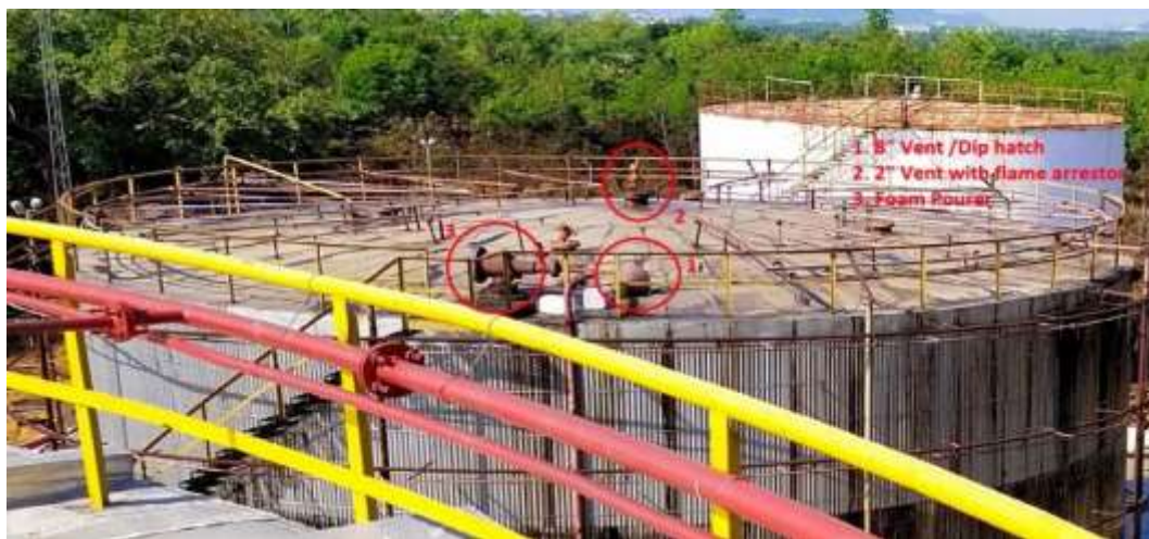
Fig 1: M6 Tank with vents on top of the tank
