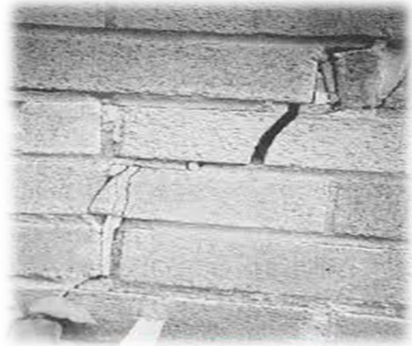
Fig. 4 Crack due to thermal movement
