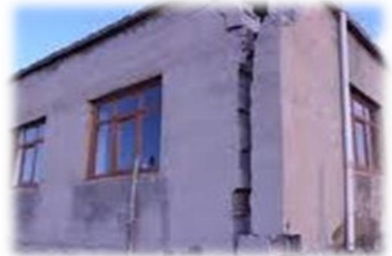
Fig. 6 Crack due to earthquake
