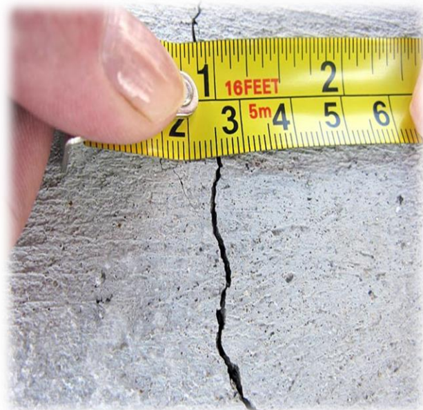
Fig. 2 Non Strctural Crack
