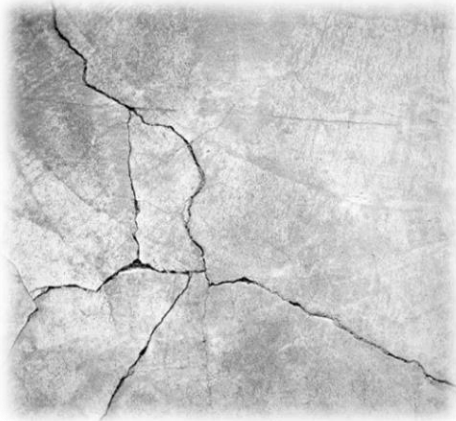
Fig. 3 Crack due to moisture change
