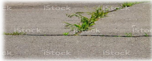
Fig. 5 Cracks due to vegetation
